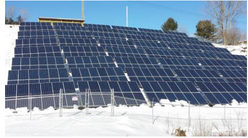
Figure 23: This is a photo of the Town-owned 150 kW solar project in Cavendish as described on page __. This is an example of a perfectly sited project. Because it is not visible from any major public roads and has no neighbors, no landscaping is warranted. (Credit: Peter LaBelle)
