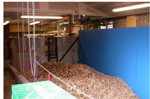
Figure 27: Wood chip heating system at Weathersfield School.
